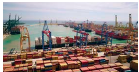
The MSC terminal at the Port of Valencia Spain has 2 x 16MW TMC transformers powering the gantry cranes.
