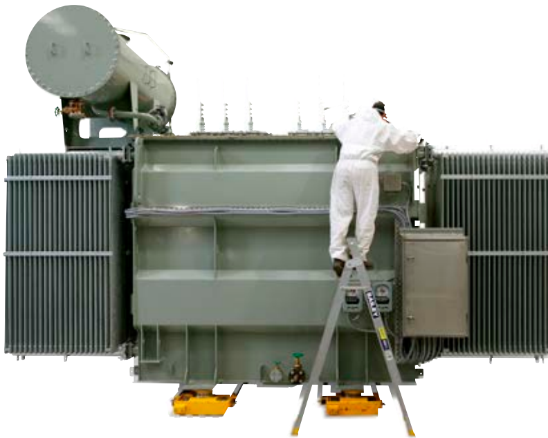
5350kVA 66000/600-600V Yy0d1 ONAN Power Transformer
