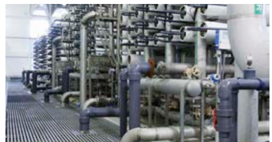
The Victorian Desalination Plant delivers up to 150 billion litres of high quality water per annum to 5 million+ residents of Melbourne Australia – around one third of the city's needs.
