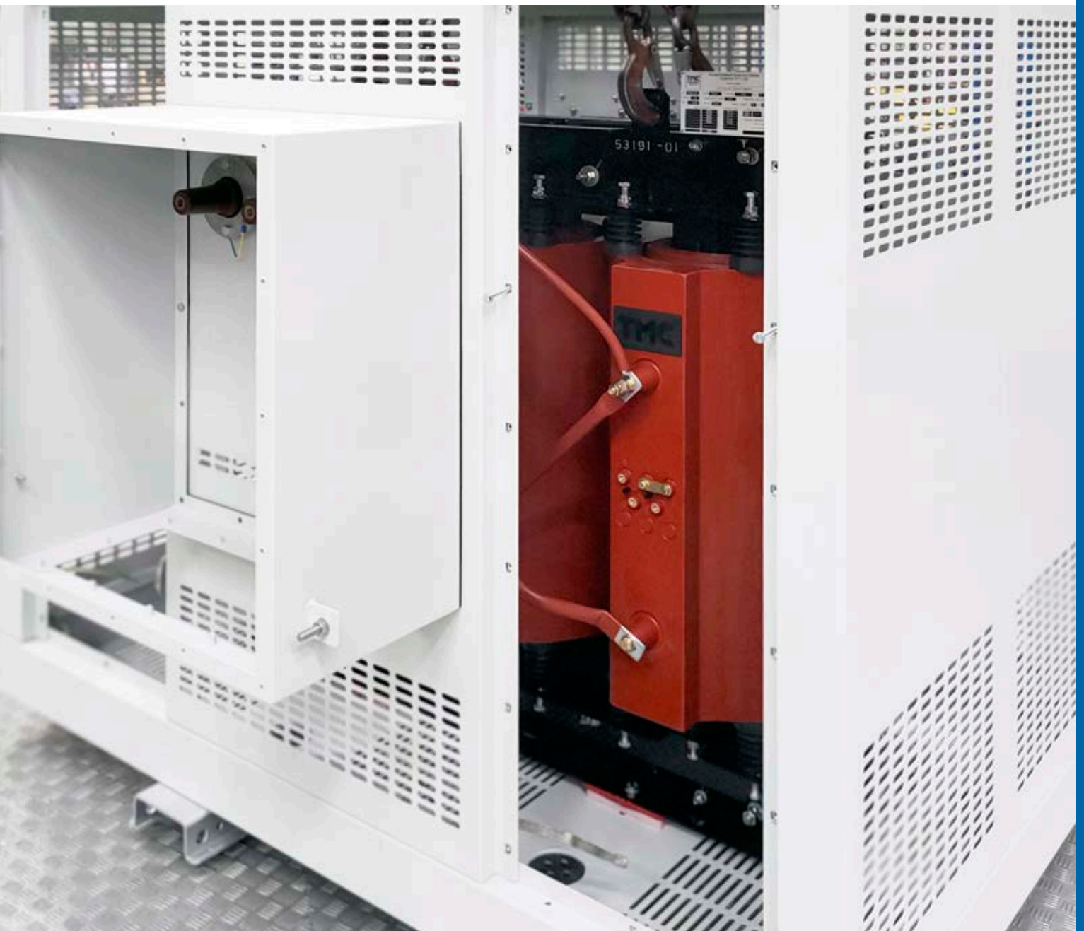
500kVA 11000/1000V AN IP21 (panels removed) with HV Cable Box and Separable Connectors
