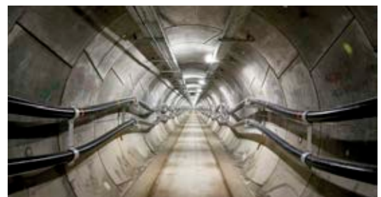
La Mat Tunnel, 8.5km high voltage tunnel running between Spain and France through the Pyrenees Mountains carrying 400kV cables for energy distribution.
