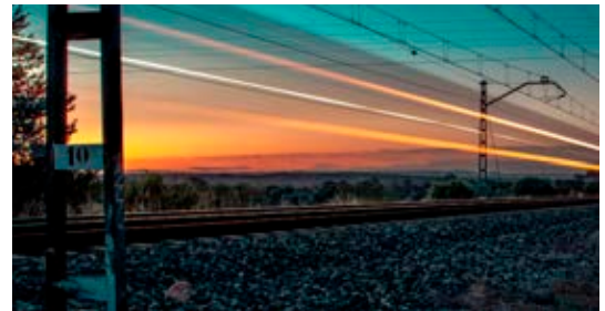
Multi-tension traction substation feeding the CAF Track test circuit in Corella, Navarra used in development and testing of passenger and freight trains.
