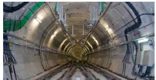
Cañizo Tunnel, Spain 5372m long servicing high speed trains connecting Madrid and Galicia.
