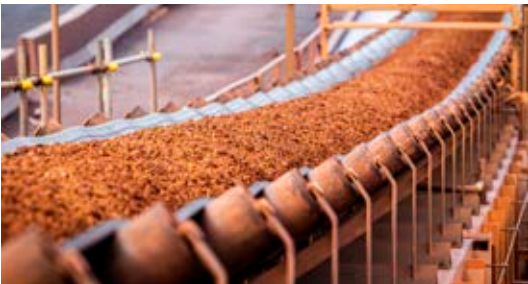
Mining conveyor belts above and below ground often in harsh environments – rough, hot, dry & salty.
